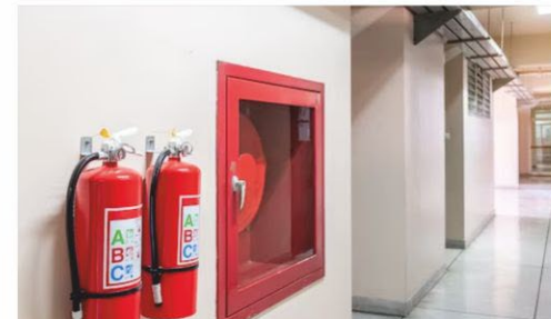
FIRE FIGHTING EQUIPMENT
